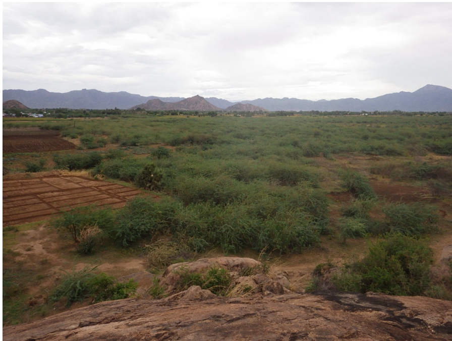
Figure A2: Invasive vegetation in tank bed highlighted tank state of disrepair.
