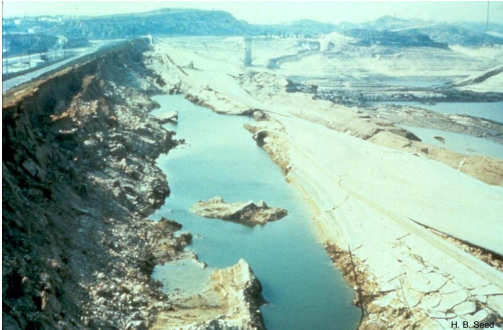
Figure 1.2 The upstream slide after liquefaction failure of Lower San Fernando dam ( http://research.engineering.ucdavis.edu/gpa/wp-content/uploads/sites/43/2015/02/Slide-after-drawdown.jpg )
