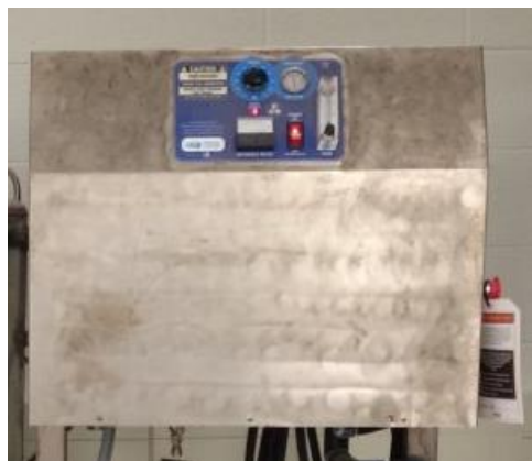
Figure 3.1 Pacific Ozone Generator
