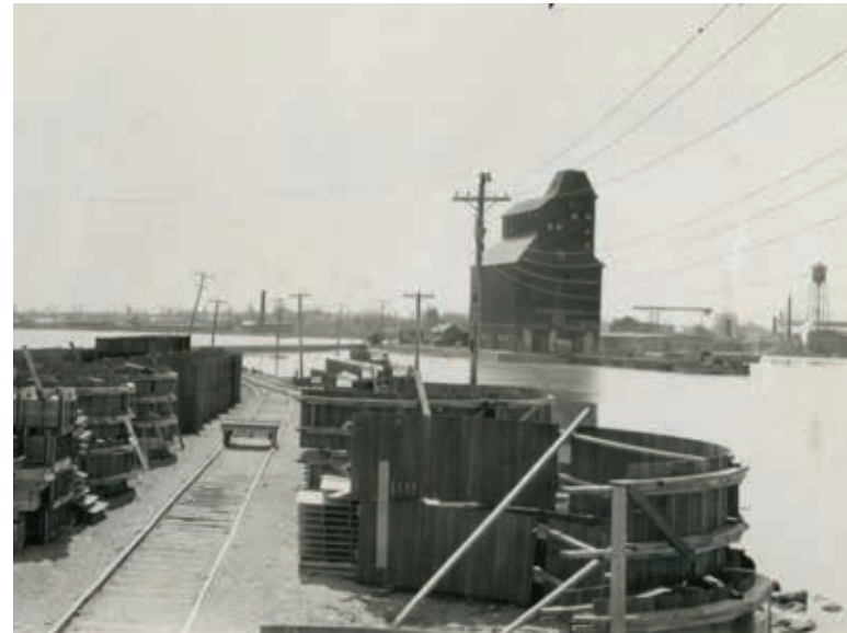
Figure 2.9 [Left] Newly materialized stockyard upon an extended Town Dock. Piles of lumber for the foundation and Work Floor concrete formwork await their use. Hastily erected huts and offices crowd the muddy edges, while the obsolete wooden elevator displays itself prominently.
