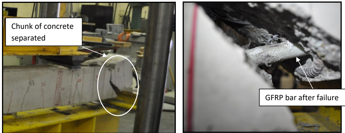
b- Beam after failure
