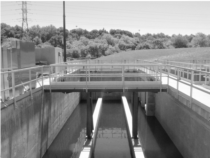
Figure.26 Filtration Process: Contact Tank
