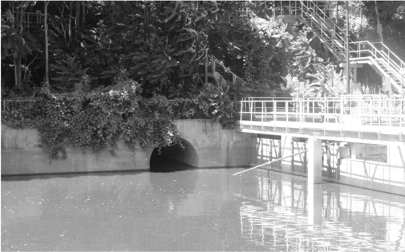
Figure.20 Filtration Process: CSO tank
