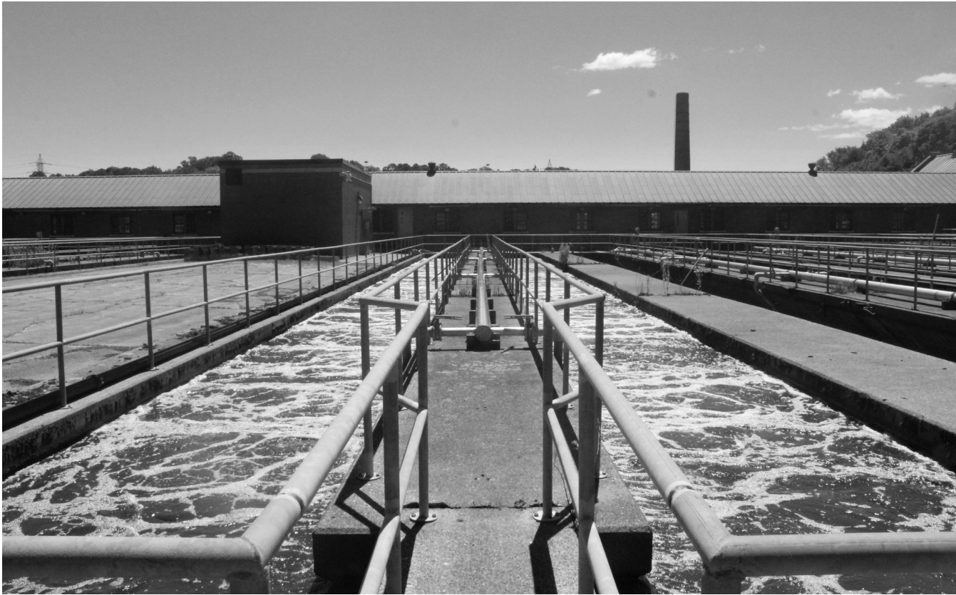
Figure.23 Filtration Process: Aeration Tanks
