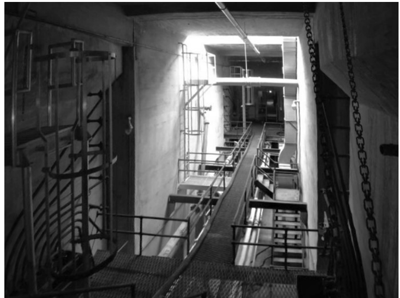
Figure.29 Filtration Process: Inside underground digestors
