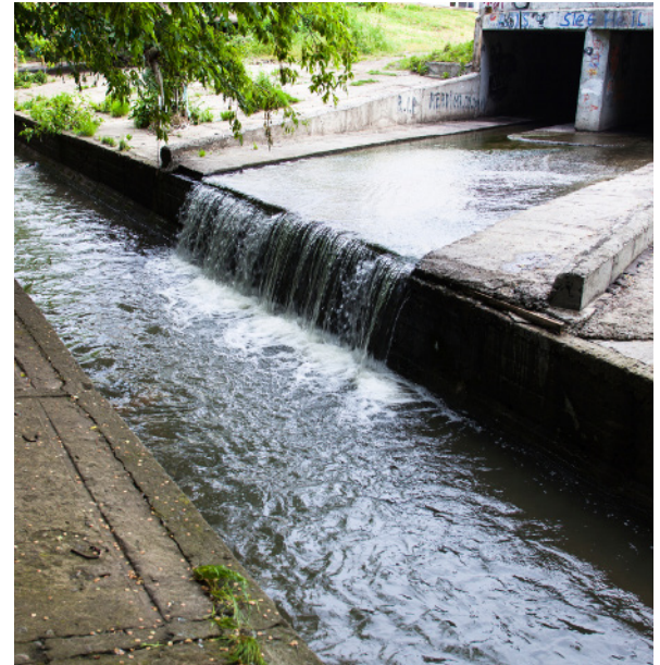
Figure.45 Waterstream from underground tunnel
