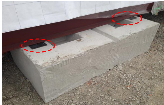
Figure 3.8. Installation of steel shims to cover the gap between modules and foundation.
