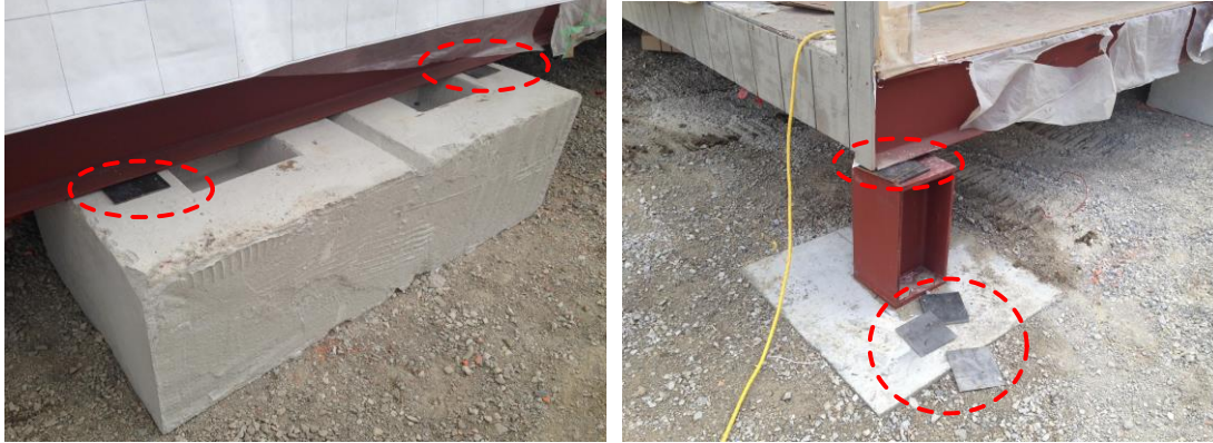
Figure 5.19. Application of steel shims to fix the excessive geometric variability issues in the bottom profile of a module during assembly processes at project site.
