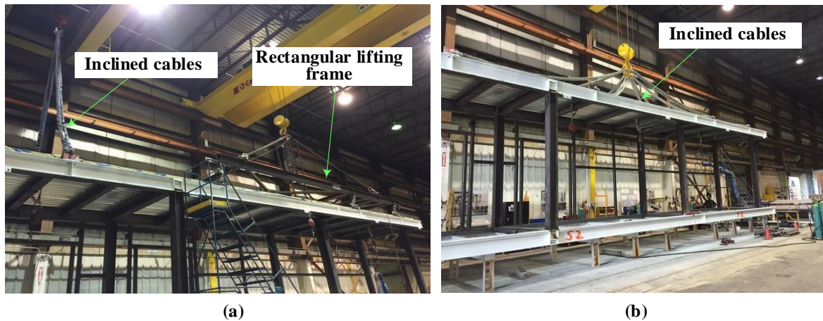
Figure 5.15. Placement of roof frame using: (a) rectangular lifting frame and inclined cables, and (b) inclined cables.
