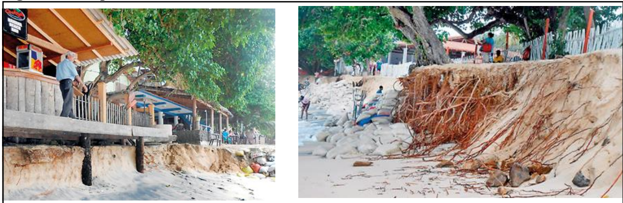
Figure 4.2: Impact of erosion on Unawatuna beach
