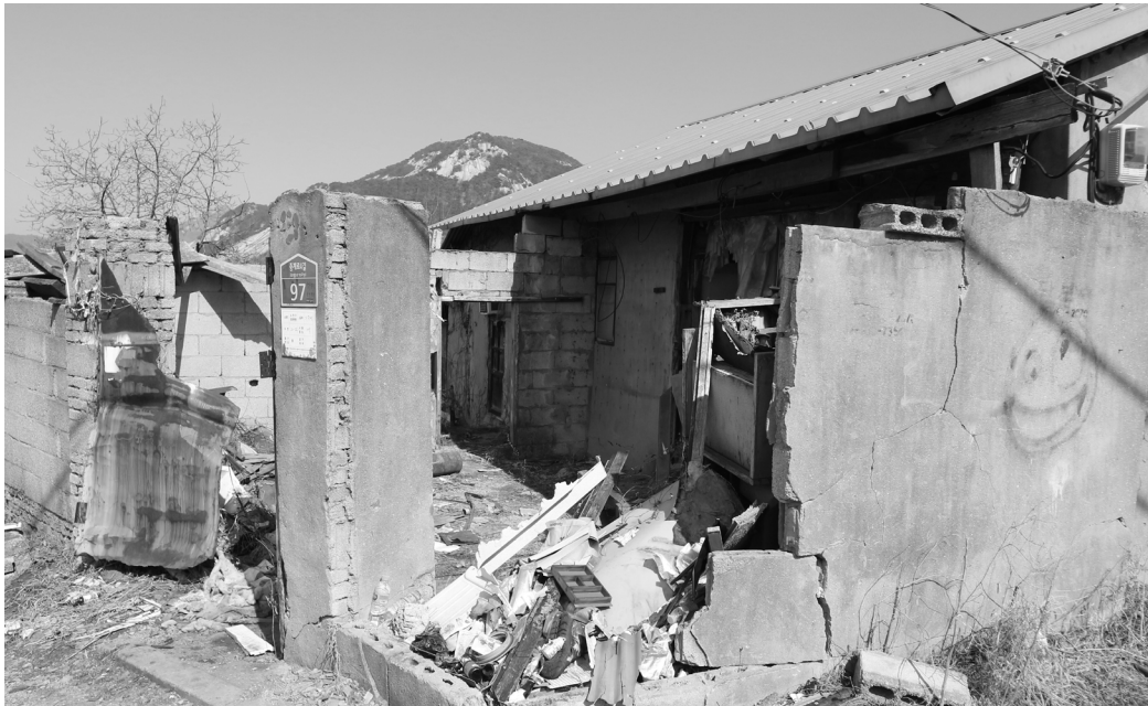
Figure 7 A Dilapidated Building in Baeksa Village
