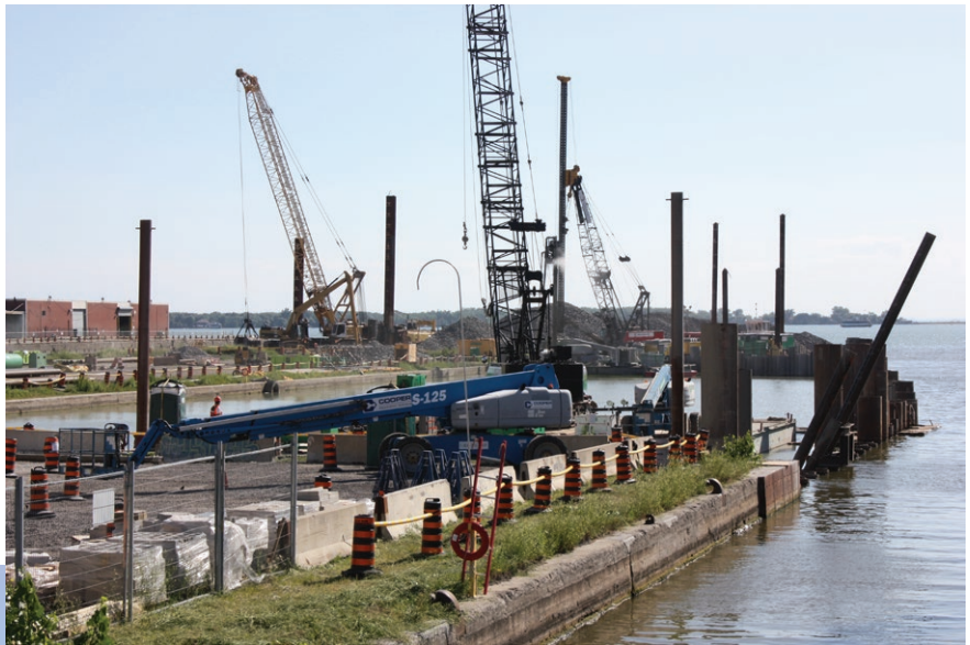
fig. 2.2 (above) Cherry Street Lake filling project begins, large cranes move new material from barges and ships into the harbour, where dump truck and bulldozer flatten and shape the new landscape.
