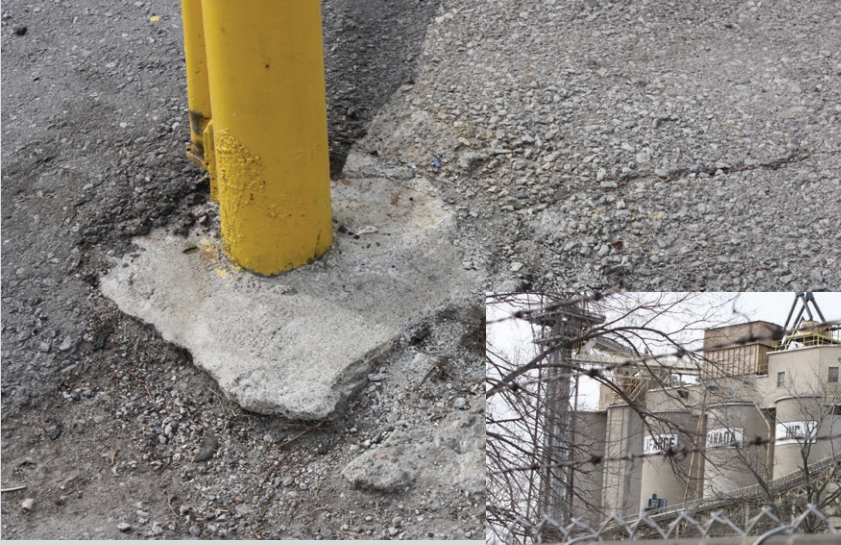
fig. 1.66 (above) layers of concrete and asphalt, punctuated by bright yellow blockades denoting caution or areas boundaries.
