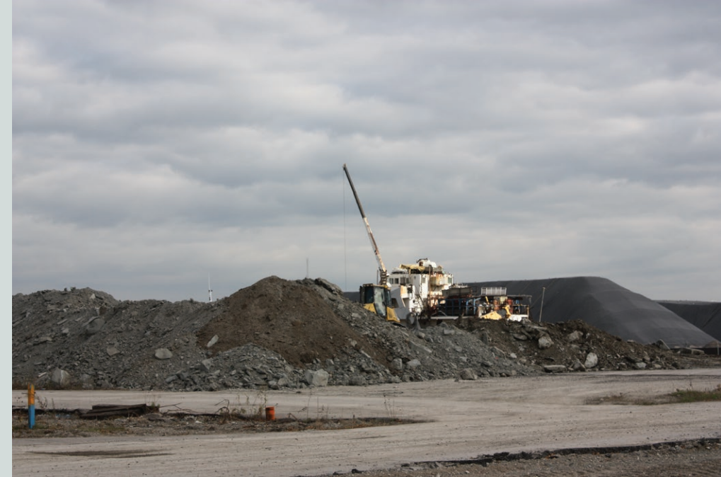
fig. 2.28 (left) Soil in the Port Lands being excavated fig. 2.29 (middle) Soil piled 20' high fig. 2.30 (right) Soil waiting to be remediated
