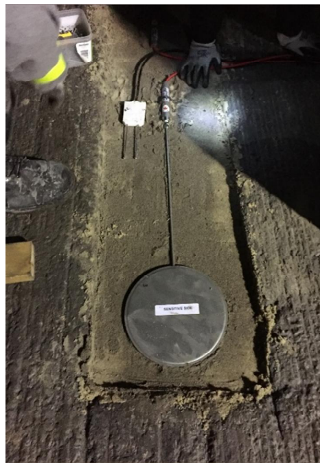
Figure 5-1. Instrumentation cluster installed underneath panels (Pickel, 2018)
