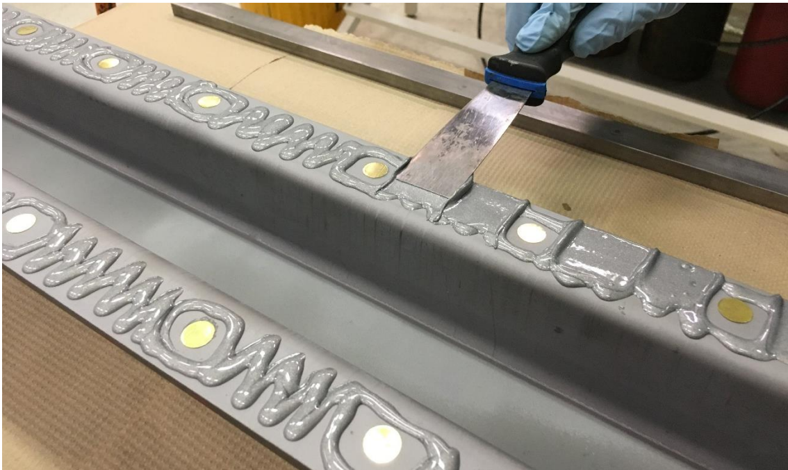
Figure 3.20: Improved shimming technique, where circular shims are used to distribute clamping forces more evenly for uniform adhesive coverage
