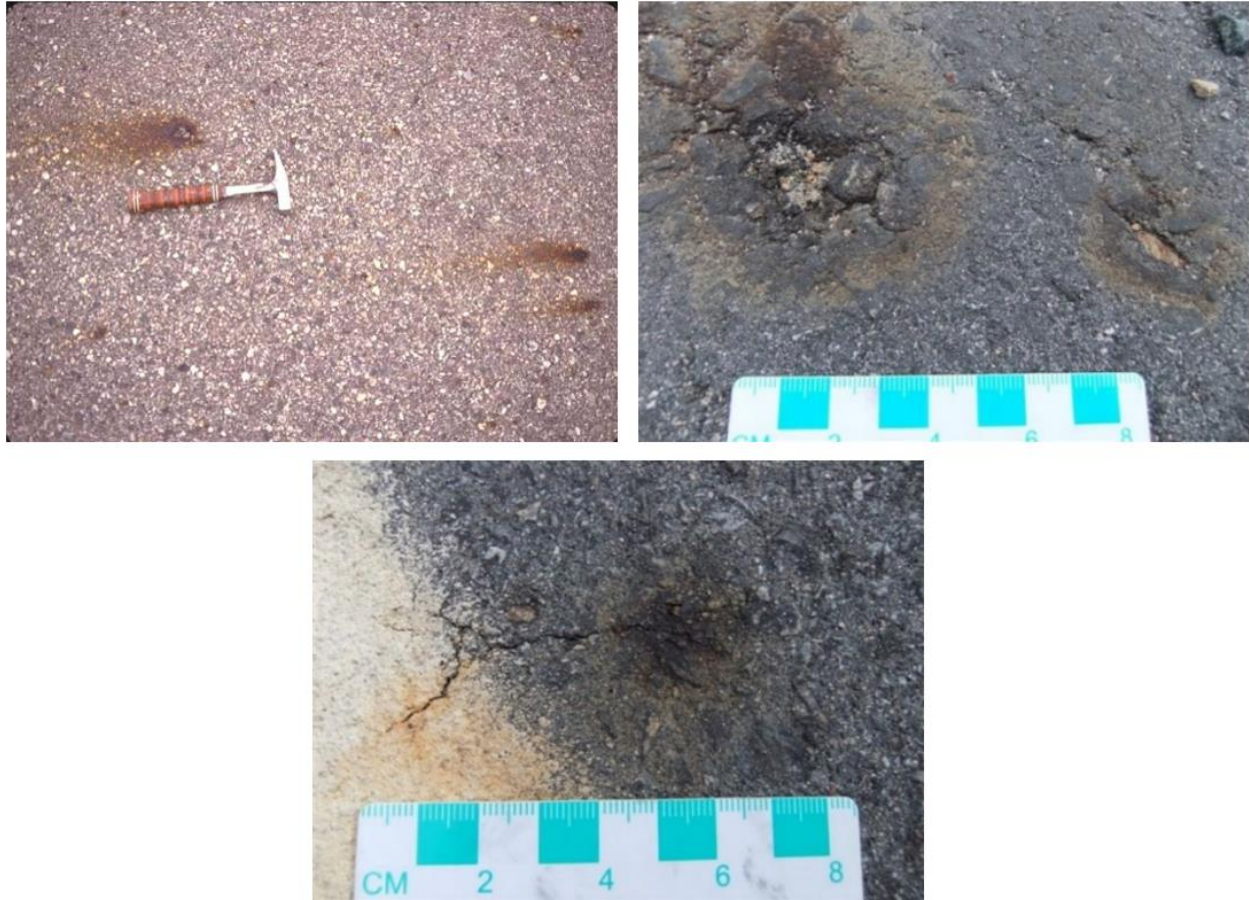
Figure 3-2 Activations of Iron Sulfide-Containing Aggregates in The Road Surface Showed Itself as Staining (Top Left), Bumping (Top Right) And Crack Initiation (Bottom)
