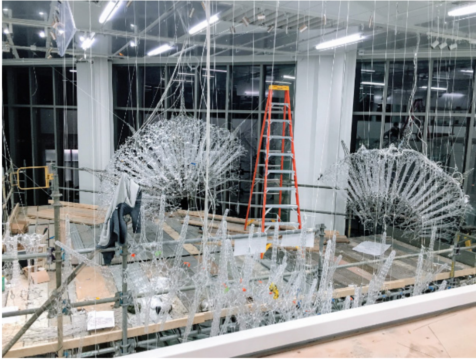
Figure 4-15: Main sphere units in place with cables adjusted to project from close to normal.
