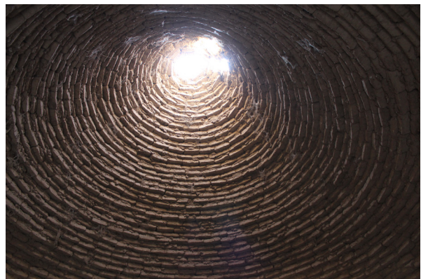
Figure 45 Traditional construction in Jazan - Dome/Vault: Earthen blocks are laid shaping curved forms that transfer compression forces to the supporting walls. To prevent rain erosion, the blocks must be fired into bricks or coated with protective finish.
