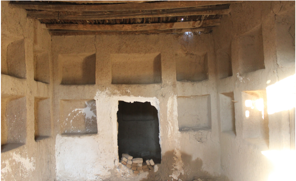
Figure 59 Abandoned house in Jazan
