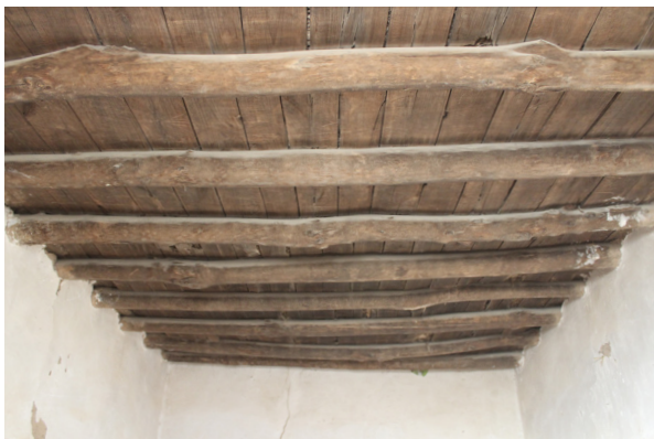
Figure 44 Traditional construction in Jazan - Flat Roofing: Beams transfer the weight of the roof to the walls. The beams are covered with wooden slabs or shubs and then coated with cob, which is extremely prone to water erosion and should be covered with more modern types of water-proofing membrane.
