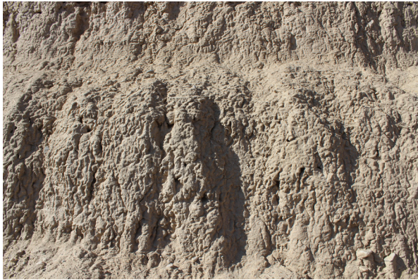
Figure 42 Traditional construction in Jazan - Wet Forming: Wet Loam is mixed with hay and processes to create cob. A team of two can then build the wall row by row, with one person sitting on the top layer and forming the next using lumps of cob handed to them by the other person.
