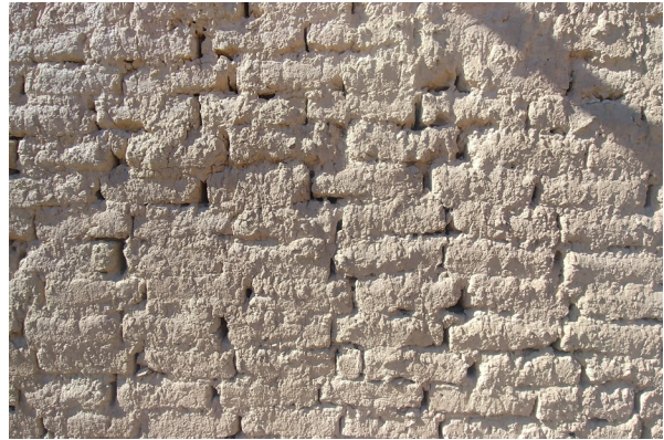
Figure 43 Traditional construction in Jazan - Adobe: Earthen blocks are formed by hand in wooden molds and dried in the sun. The blocks are then laid to form the wall with mortar in horizontal and vertical joints. A coating of cob may be applied as the finish layer.
