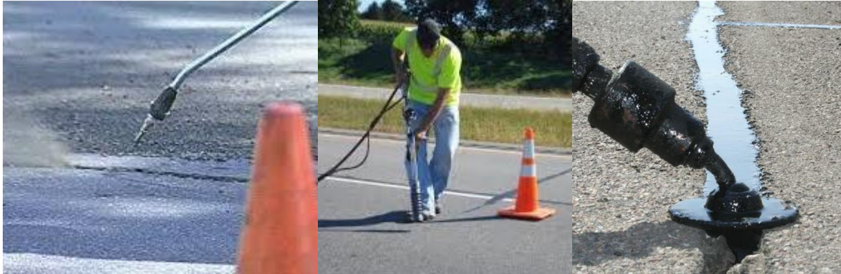
Figure 3.1: Left – Crack Cleaning With Compressed Air (Decker 2016), Centre – Hot Air Lance (Al-Qadi, Imad L Ozer et al. 2016), Right – Crack Sealant Application (AsphaltPro 2019)
