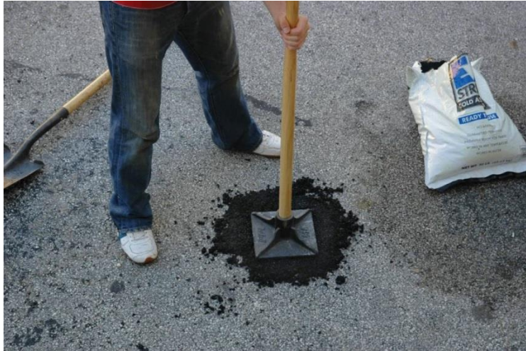
Figure 3.5: Pothole Repair Using Cold Mix Asphalt and Hand Tamper for Compaction (EZ Street Asphalt 2019)
