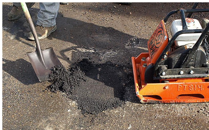
Figure 3.4: Hot Mix Asphalt Pothole Repair Using Plate Tamper for Compaction (City of Edmonton 2019)
