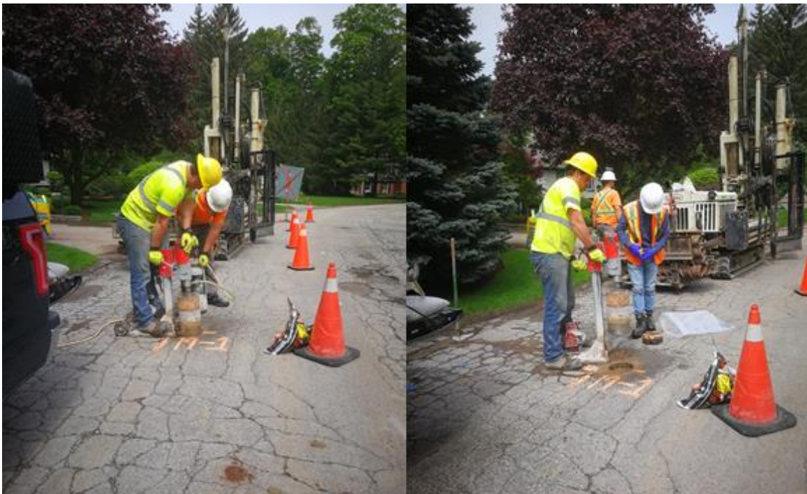
Figure 4.17: Left – Drilling Asphalt Core BH19-1, Right – Retrieving Asphalt Core BH19-1, Taken May 30 th , 2019
