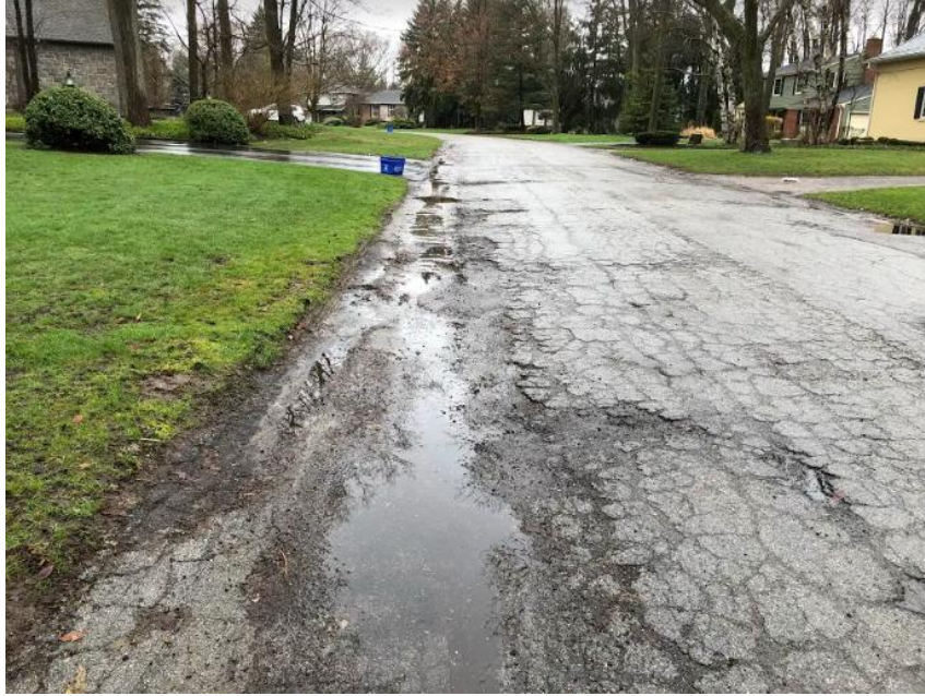
Figure 4.5: Pavement Distortion Along Sides of Sugarbush Drive, Taken May 8 th , 2019
