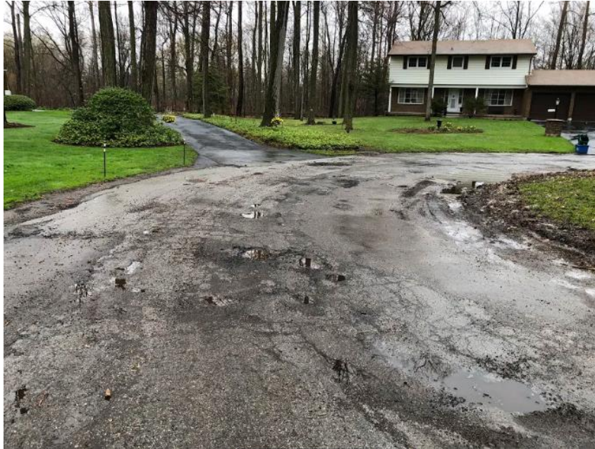
Figure 4.3: Potholes and Cracking Around Curve in Sugarbush Drive, Taken May 8 th , 2019
