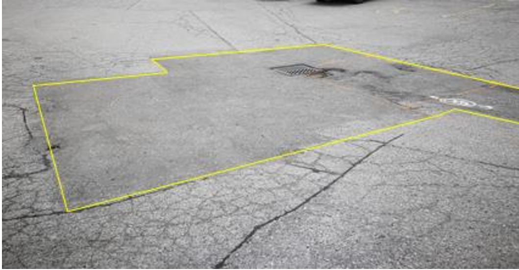
Figure 3.10: Storm Drain Region with Two Year Old Patch Marked for Repair
