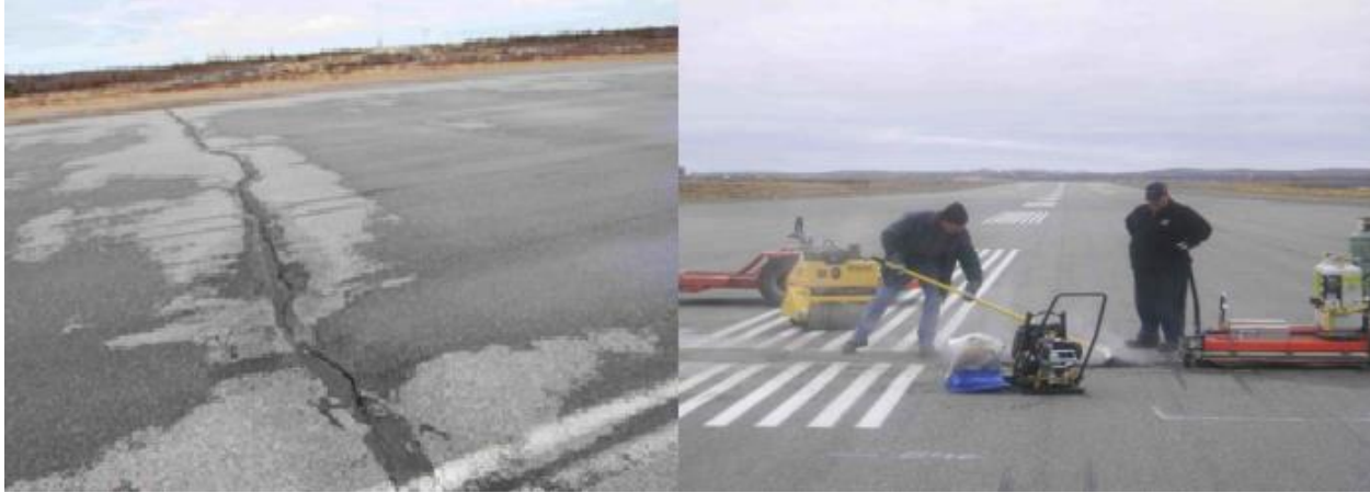
Figure 2.4: Kuujuuaq Airport. Left: Crack Before Repairs; Right: Crack During Infrared Heating Repairs (Kieswetter 2013)
