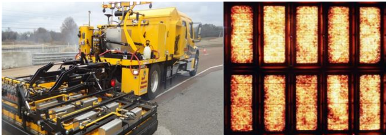
Figure 1.1: Left: Infrared Heating Machine in Use, Right: Bottom of Machine in Use (Kieswetter 2013)
