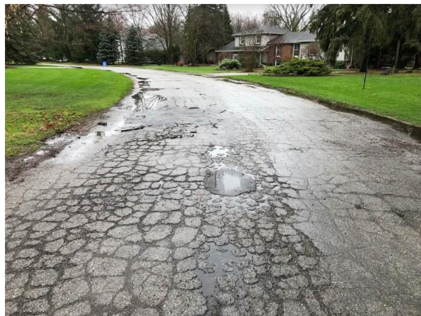
Figure 4.4: Block Cracking, Potholes, and Drainage Issues, Taken May 8 th , 2019
