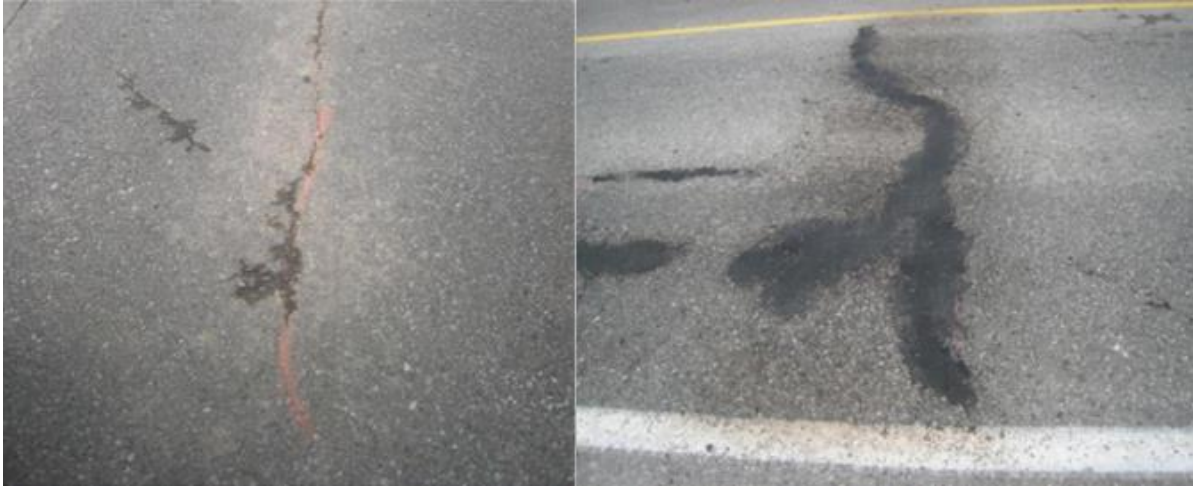
Figure 2.3: Left – Cracking on Bleams Road; Right – Repaired Cracking on Bleams Road (Uzarowski et al. 2011)
