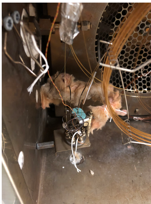
Figure 7.11 Insulated copper tubing for compressed airline.
