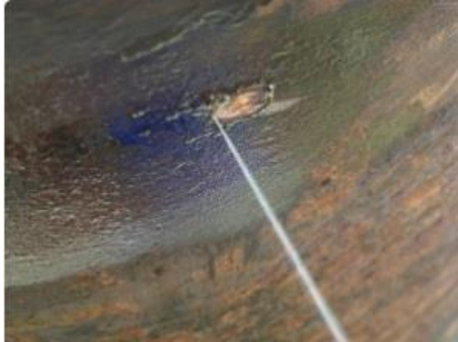
Figure 2.1 Example of a pinhole leak [2].
