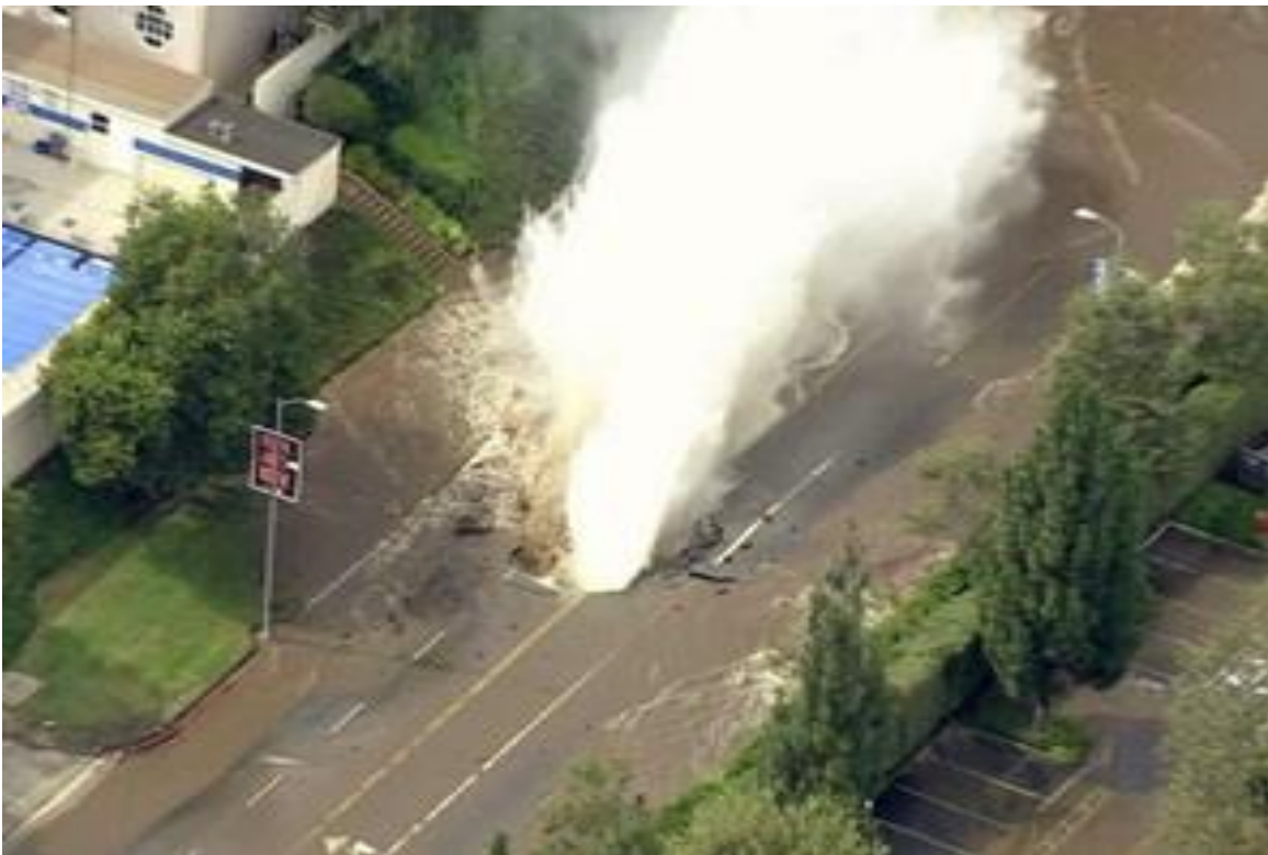
Figure 1.1 Water burst resulting in damage to a road [1]
