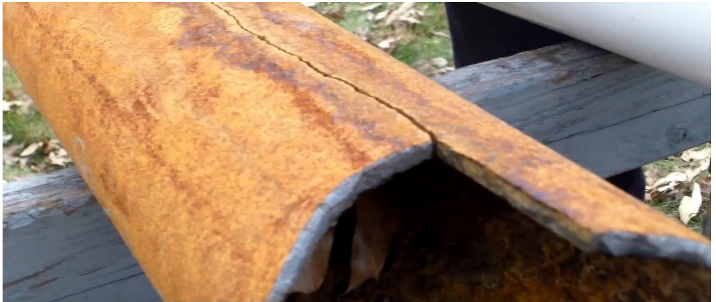
Figure 2.2 Example of a cracks in the pipes which can result in large leaks [3].
