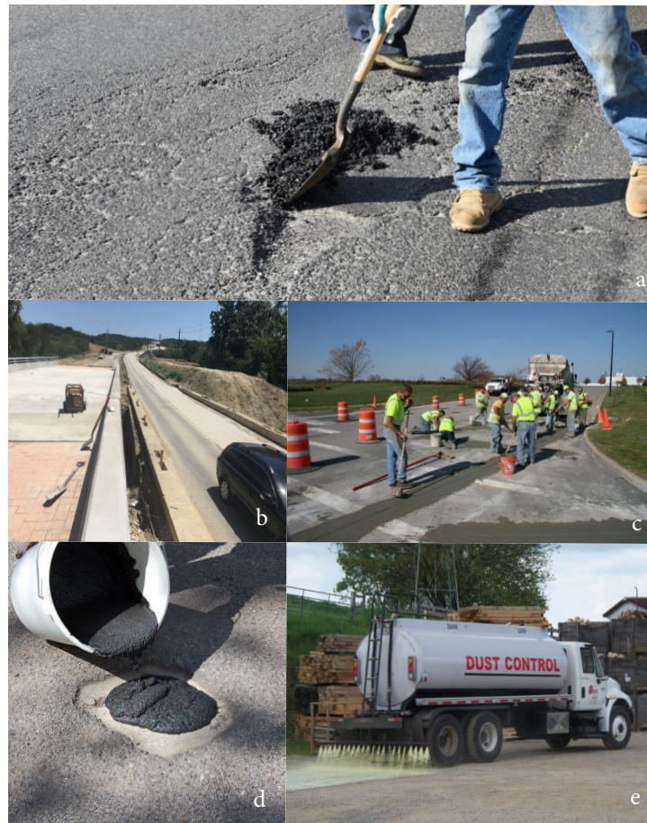
Figure (2.3) Roadway Maintenance Activities 1 a: Pothole Repair on Flexible Pavement; b: Drainage Improvement on Rigid Pavement; c: Partial-depth Slab Repair; d: Shallow Patching on Thin Bituminous Surfaces; e: Dust Control on Gravel Roads
