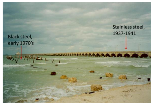
Figure 2-1. Pier in Progreso, Mexico built with 304L stainless steel and carbon (black) steel [29].
