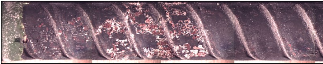
Figure 4.2-18: Example of corroded rebar on specimen 26 from NaCl SEPS
