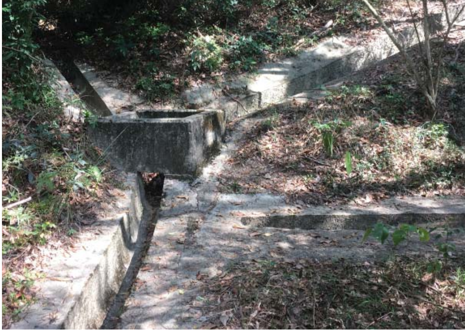
Figure 4.13 Concrete U-channels and catchment pit
