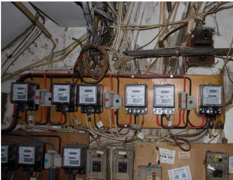
Figure 2.9 Unorganized Electrical Panel for Subdivided Units
