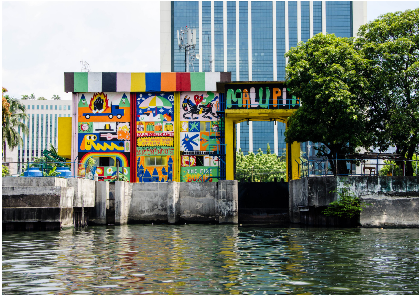
fig. 3.30 Makati Pumping Station. Makati.
