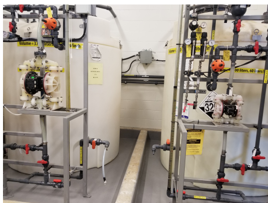
Figure 2.3: Invasive chemicals set next to each other in chemical oxidation room
