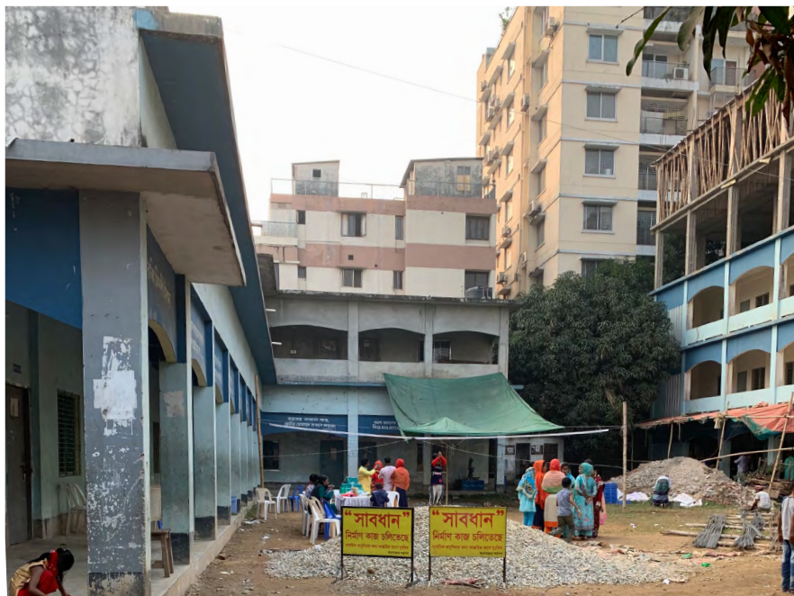
Figure 5.60: Construction material is seen to have taken over the school's playground.
