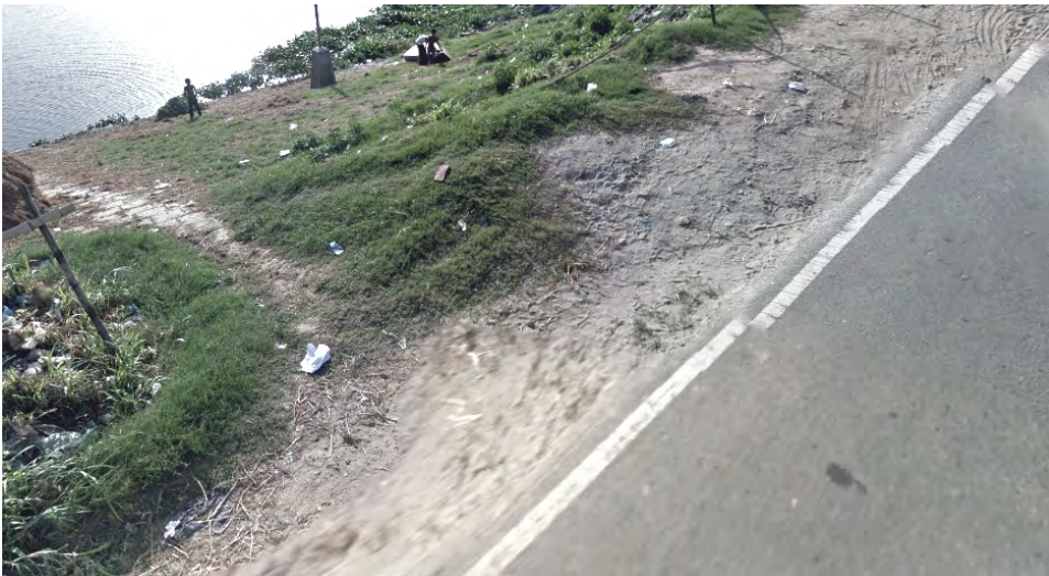
Figure 1.23: The slope of the embankment along Buriganga river is protected by concrete block.
