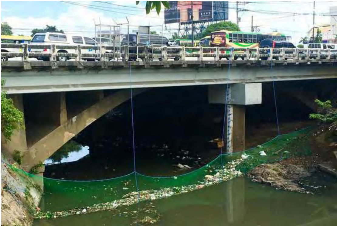
Figure 5.47: Trash trap used in San Juan River in Manila. Similar net will be proposed to be used in this design.
