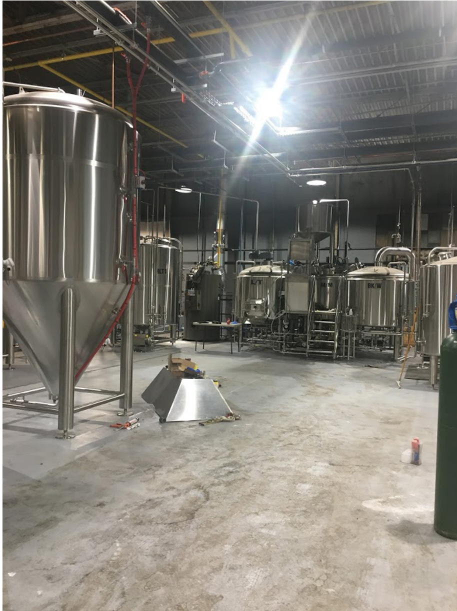
fig.0.4. Four Fathers Brewery Under Construction Adaptive Reuse of former Simplicity washing machine factory, in Hespeler, Ontario
