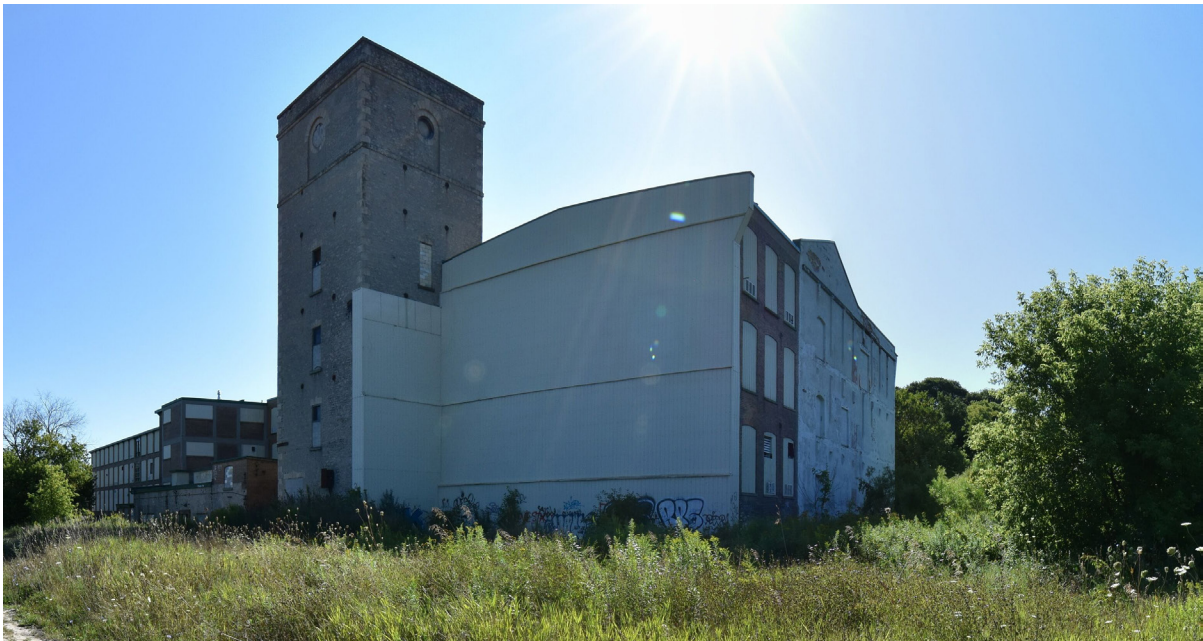
fig.3.53. Photograph of Mill no.2 Covered in Metal Siding after the Fire
