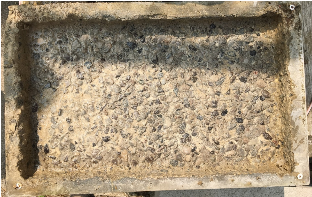
Figure 4-8: Ponding well of outdoor specimens exposed to multi chloride brine for more then 3 years
