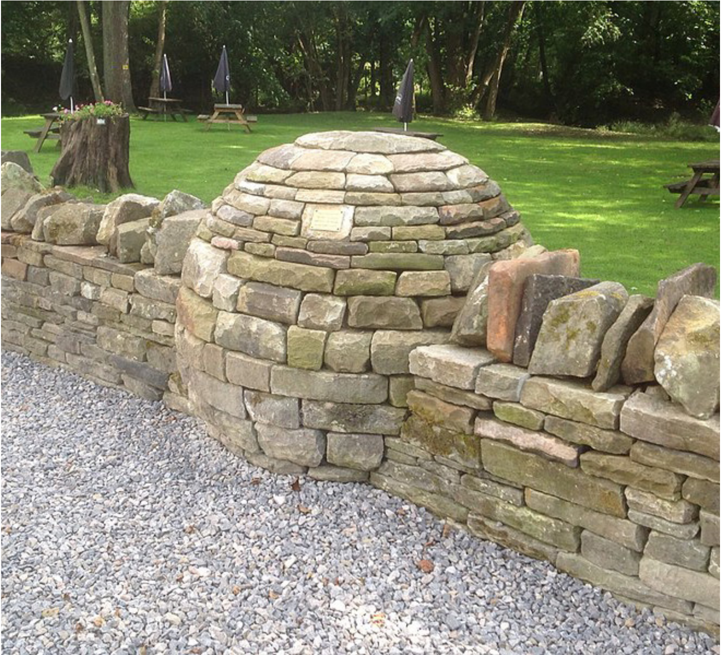
F.72. The assembly system of a dry-stacked stone wall can be used for stacking reclaimed rubble.
