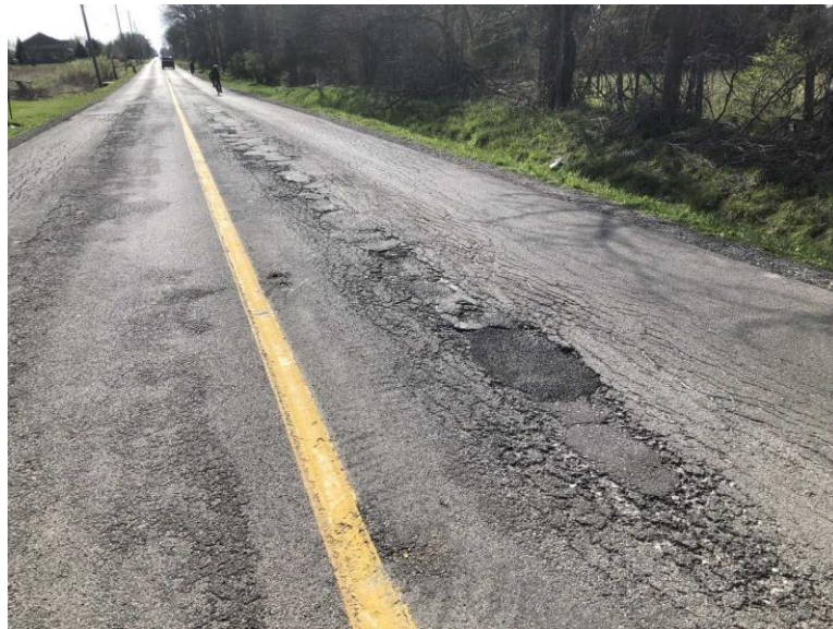
Figure 1-1: Severe Pavement Distress
