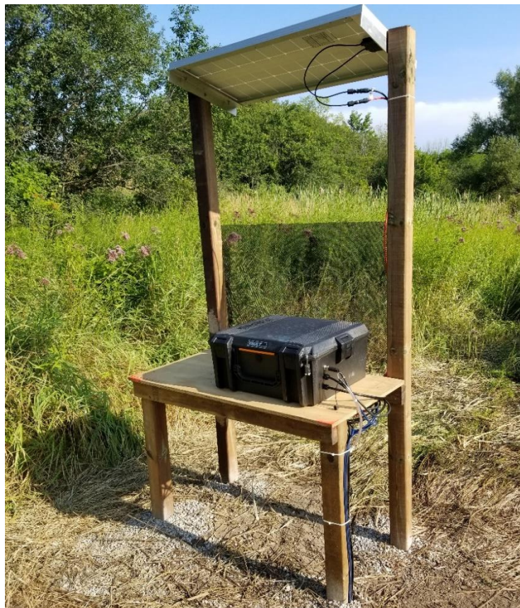
Figure 16. Electronics enclosure mounted to tabletop frame. Figure shows early version of station setup with only one solar panel.
