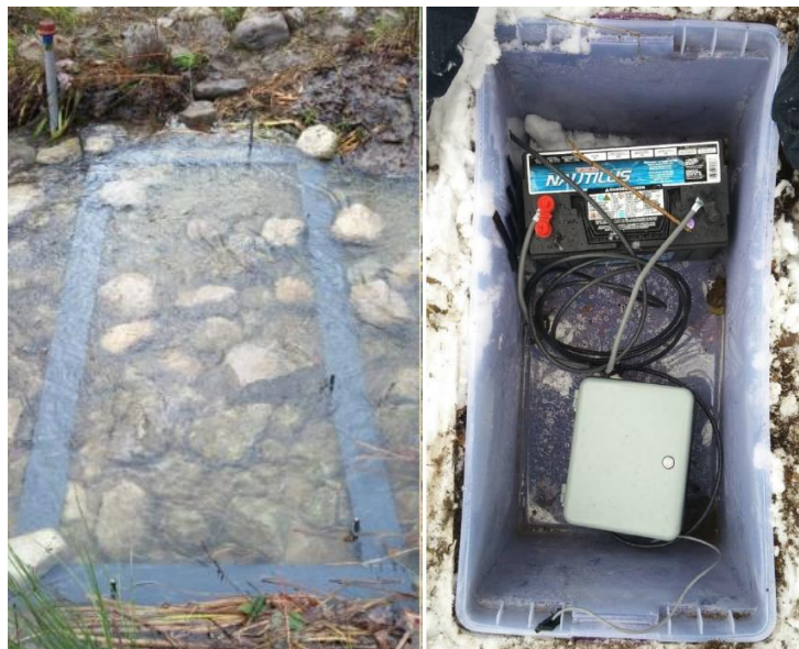
Figure 14. Muirhead Station water level gauge and in-stream antenna (left), and electrical components housed within a storage bin (right) at Schneider Creek. From (Muirhead, 2018).
