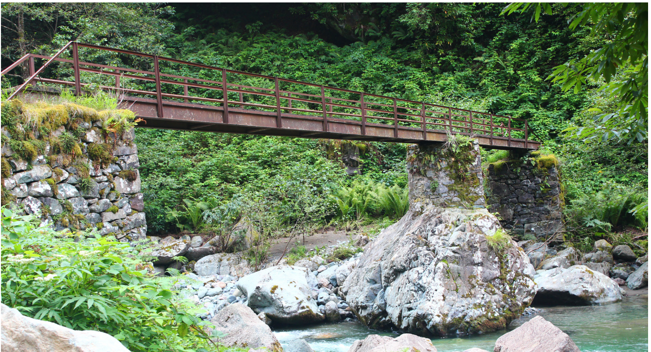
Figure 2.22 Steel bridge. This image is a reminder of the constant struggle against nature in Black Sea Region, infrastructure upkeep is a constant requirement through centuries. Original masonry bridge was repaired with a steel addition. Eastern Black Sea Mountains. © Ilhan Gokay Ozdemir.
