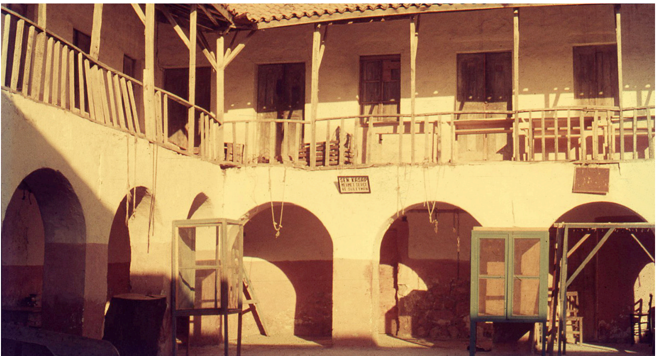
Figure 4.19 An open hayat building in Bodrum. The signs and various furniture on the ground level suggest that it was used for commercial functions (butcher shop, bakery, etc.). Upper level might have been kept as residential quarters. Photograph by Cengiz Bektas, SALT Research.
