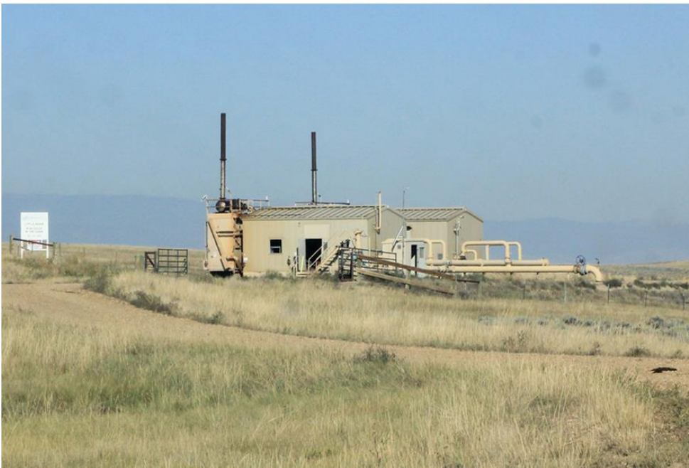
Figure A6. Compressor station.
