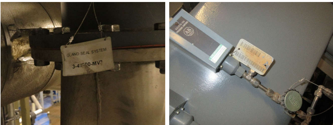
Figure 6.11 Instances where Equipment ID tags are not detected due to damage to the object itself (a) IMG_1167.JPG shows damage to the text and (b) IMG_1242.JPG shows discoloration
