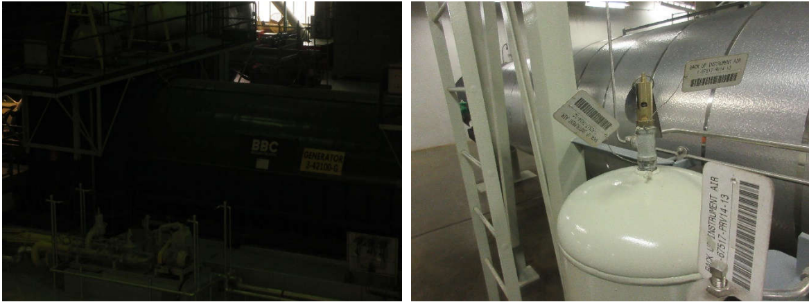
Figure 6.10 Undetected Equipment ID tags due to lighting (a) IMG_1288.JPG and (b) IMG_1247.JPG
