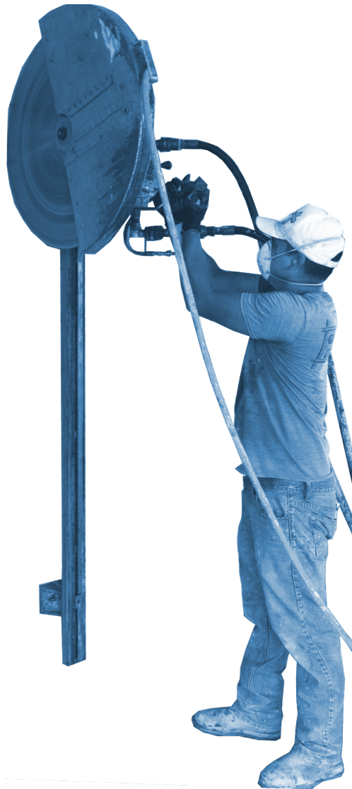
Figure 34 Wall sawing is one of the most effective ways to create openings during selective demolition. (True-Line Cut'n Core, 2020)
