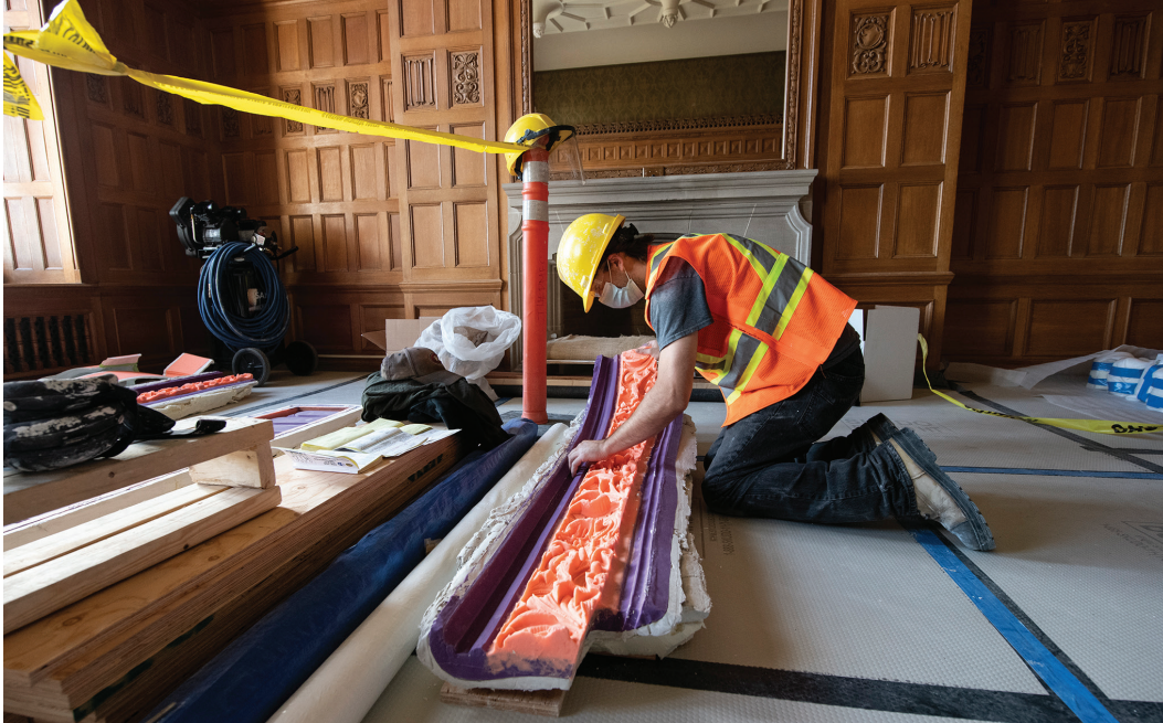
Figure 28 A plaster specialist makes a silicone mold of plaster friezes in the Senate suite in September 2020
