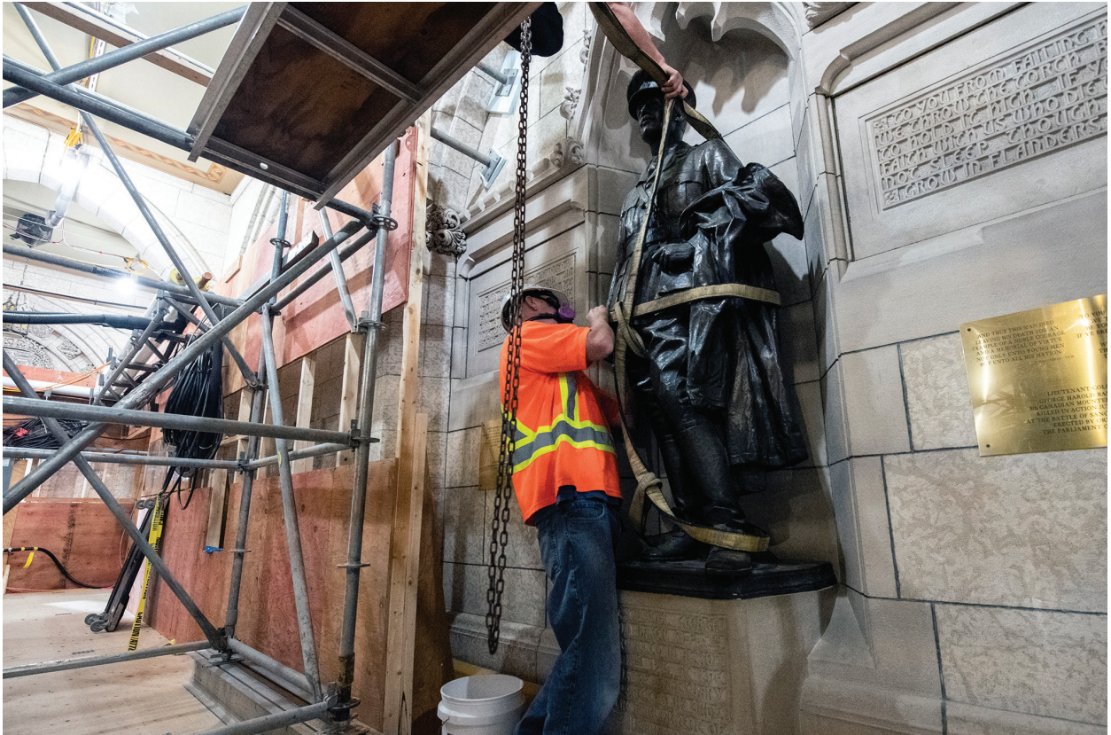
Figure 25 Workers are removing the Baker Memorial from the House of Commons foyer
