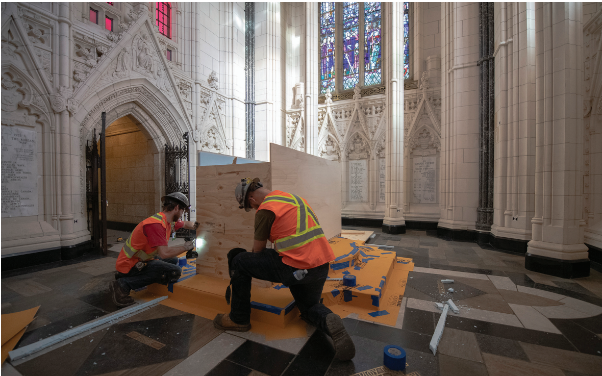
Figure 52 Workers install plywood to protect the First World War altar in the Memorial Chamber
