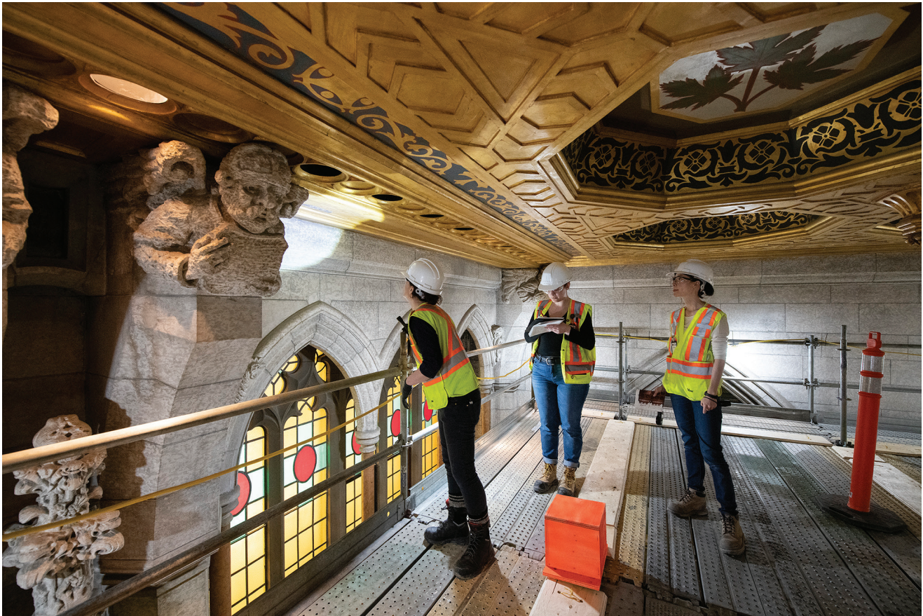
Figure 32 Workers assess the condition of the ceiling of the Senate Chamber in February 2020
