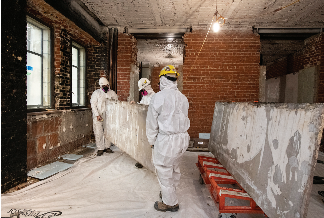
Figure 21 Workers remove decorative marble slabs from the wall of a room in the Centre Block
