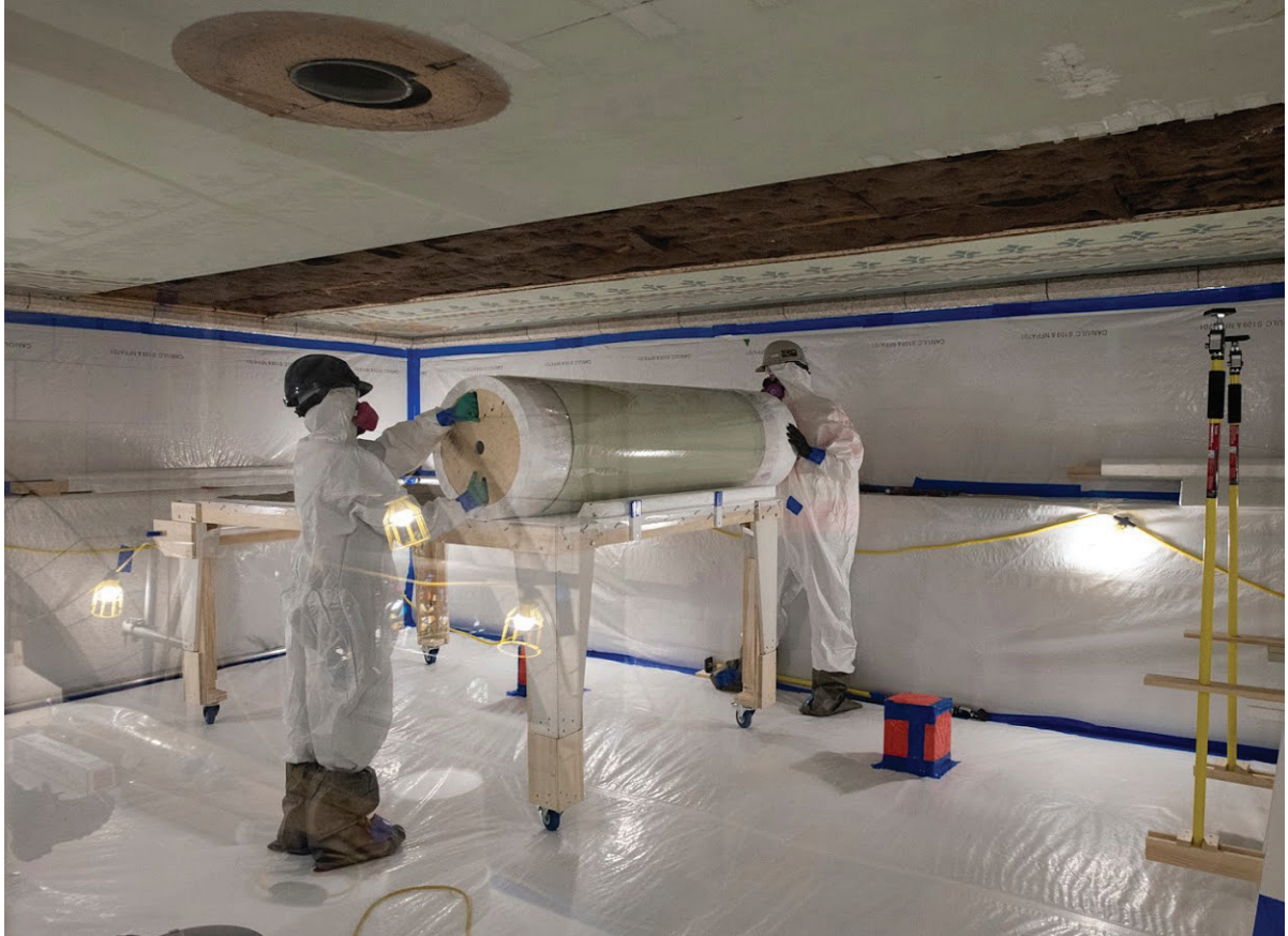
Figure 36 Two workers wearing protective equipment remove painted fabric from a ceiling and wind it onto a large spool
