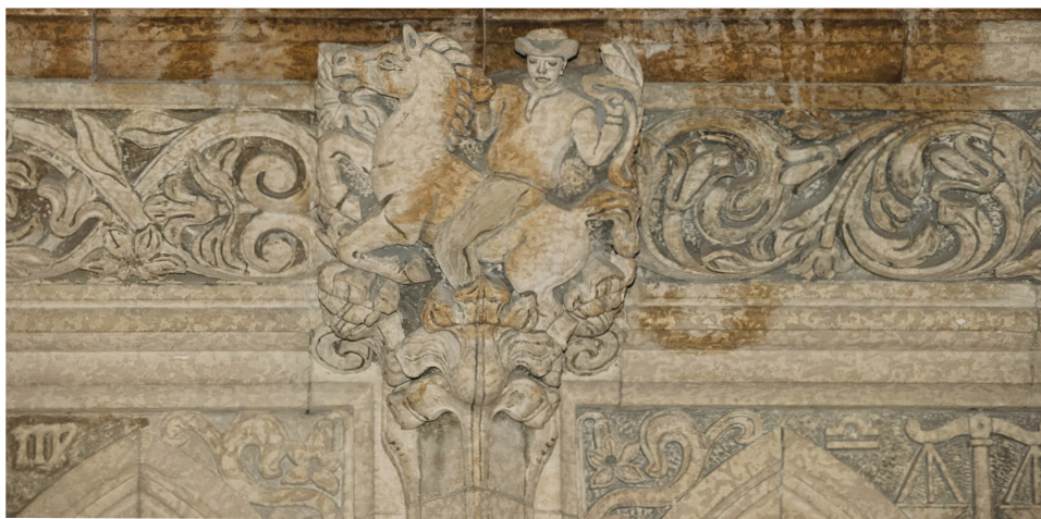
Figure 26 Some stone carvings are damaged by water leaks
