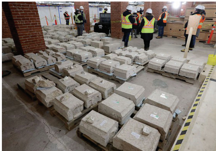
Figure 22 Interior stone blocks, each one tagged, are seen at the construction site
