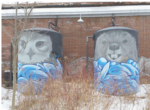
4.8 _ Rainwater Cisterns for Gardening And Flushing
