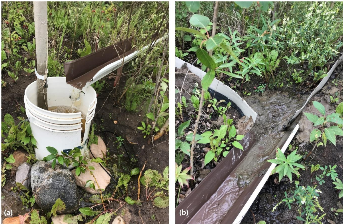
Figure 2-4 Runoff flume installed on the east slope. (a) one end of the flume was instrumented with sample bottle attached to collect runoff water sample. A pressure transducer installed in the bucket was used to estimate flow. (b) flow-collector above the flume, sealed with hydraulic cement.
