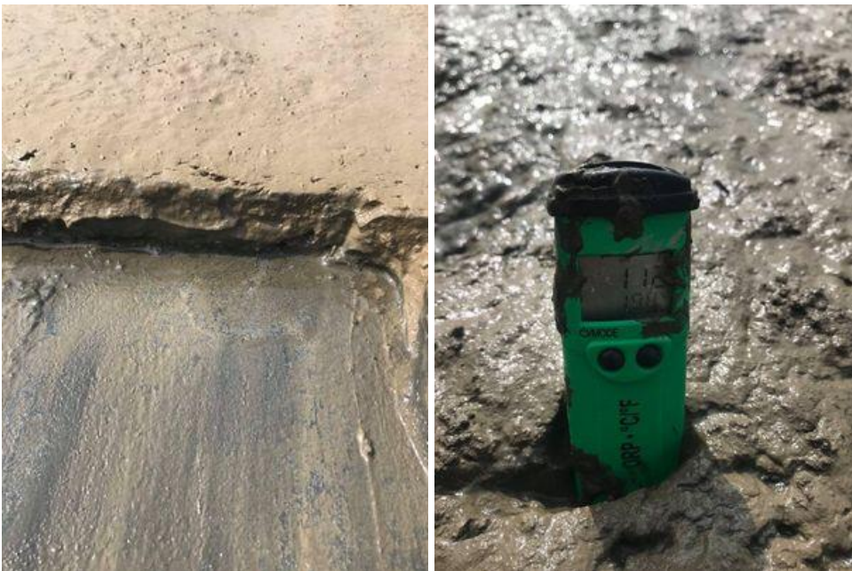
Figure G2: Sediment accumulated on the reservoir floor, along with an example of ORP probe in use.
