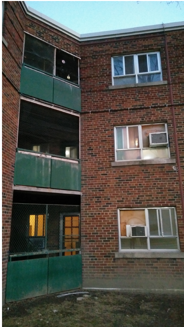
Fig. 5.34 The deteriorating conditions of the housing stock at Regent Park
