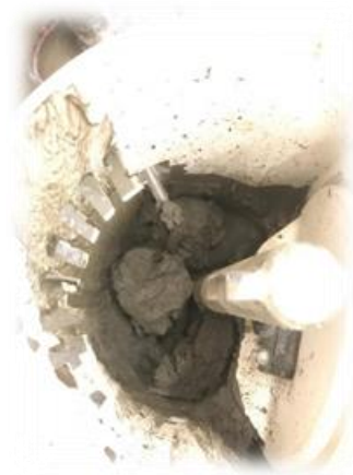
Figure 3-20, The clogged wet chamber WC0.36SP0.0
