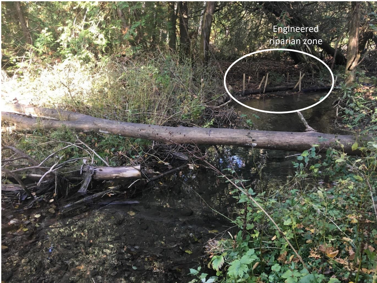
Figure 5. Washington Creek has been restored in some areas including meanders where engineered riparian zones (circled) have been built. These areas are composed of sticks, logs, and stakes to restore fish habitat and prevent erosion.
