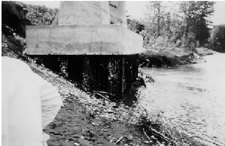
Figure 1.1: Scoured bridge foundation (MTO 1997)
