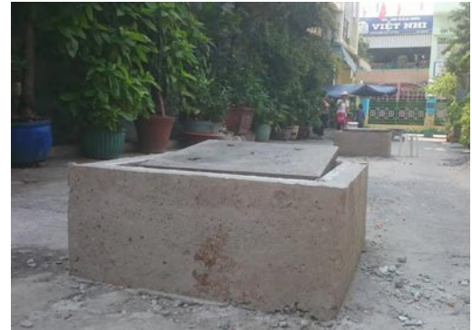
Fig. 2.10 The height of this manhole indicates where the elevated alleyway's new level will be.
