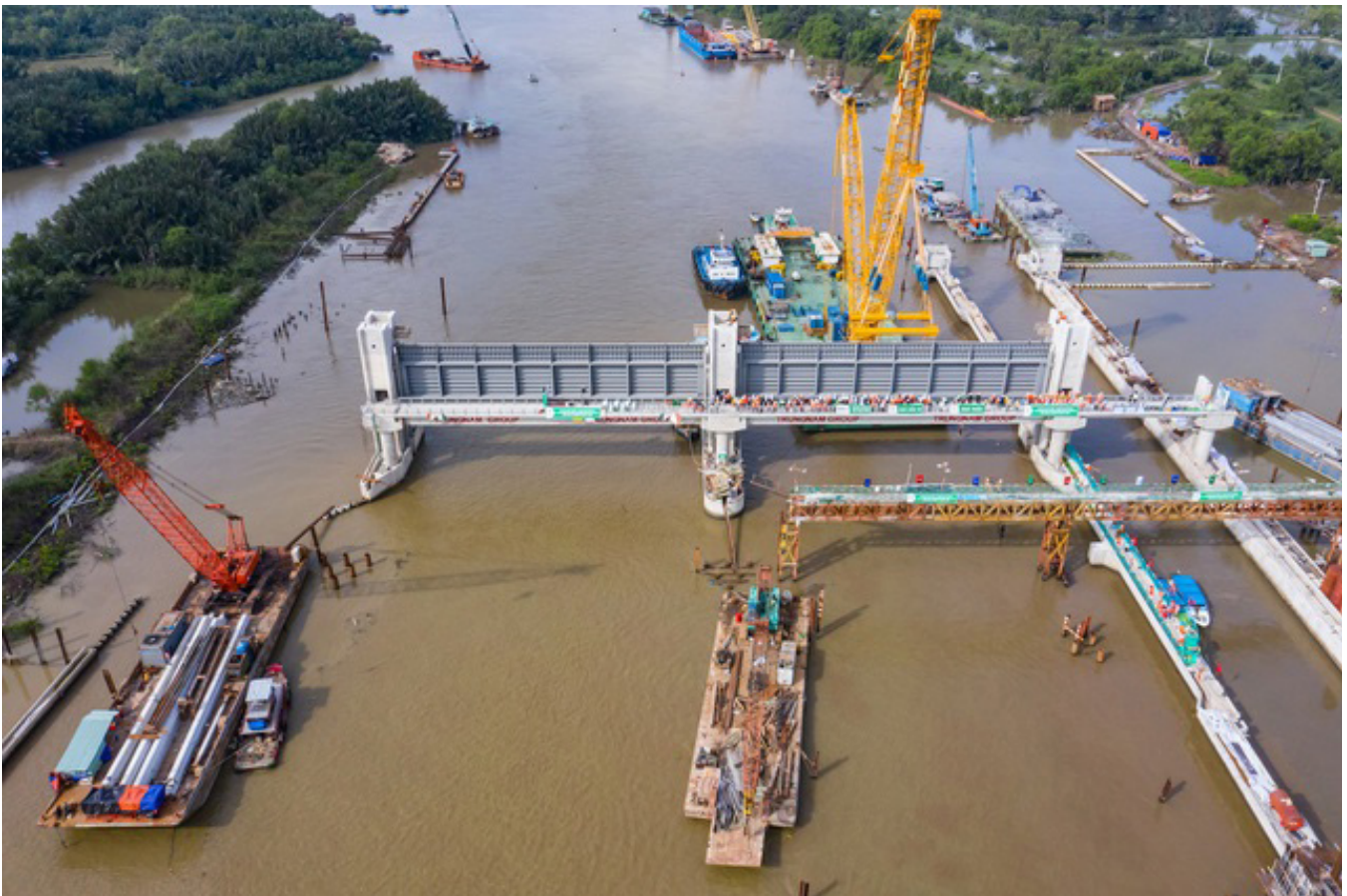
Fig. 3.21 Cay-Kho flood gate (1 of the 12 flood gates). 2021.
