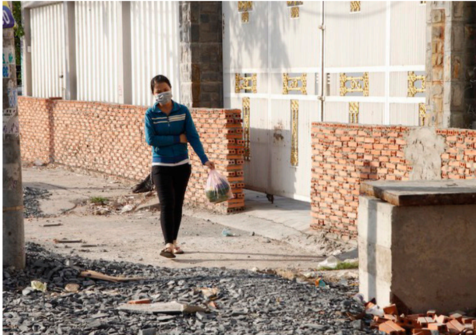
Fig. 2.13 Retaining brick walls being built to respond to the elevation of a street.
