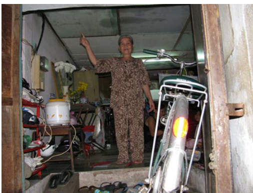
Fig. 2.09 A house that has a very low ceiling due to elevated ground floor.
