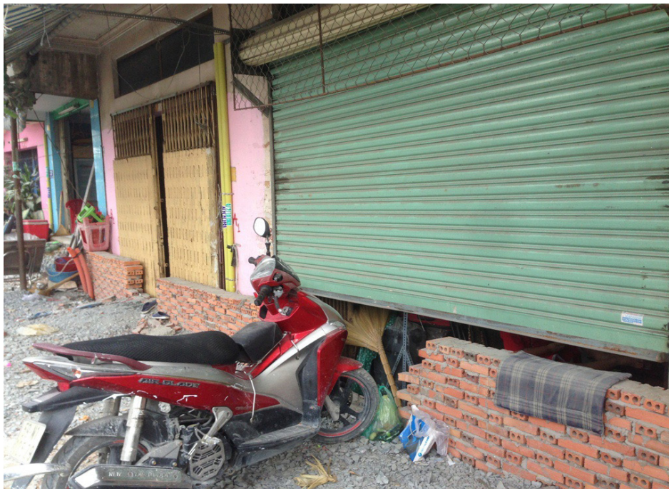
Fig. 2.14 Retaining brick walls being built to respond to the elevation of a street.
