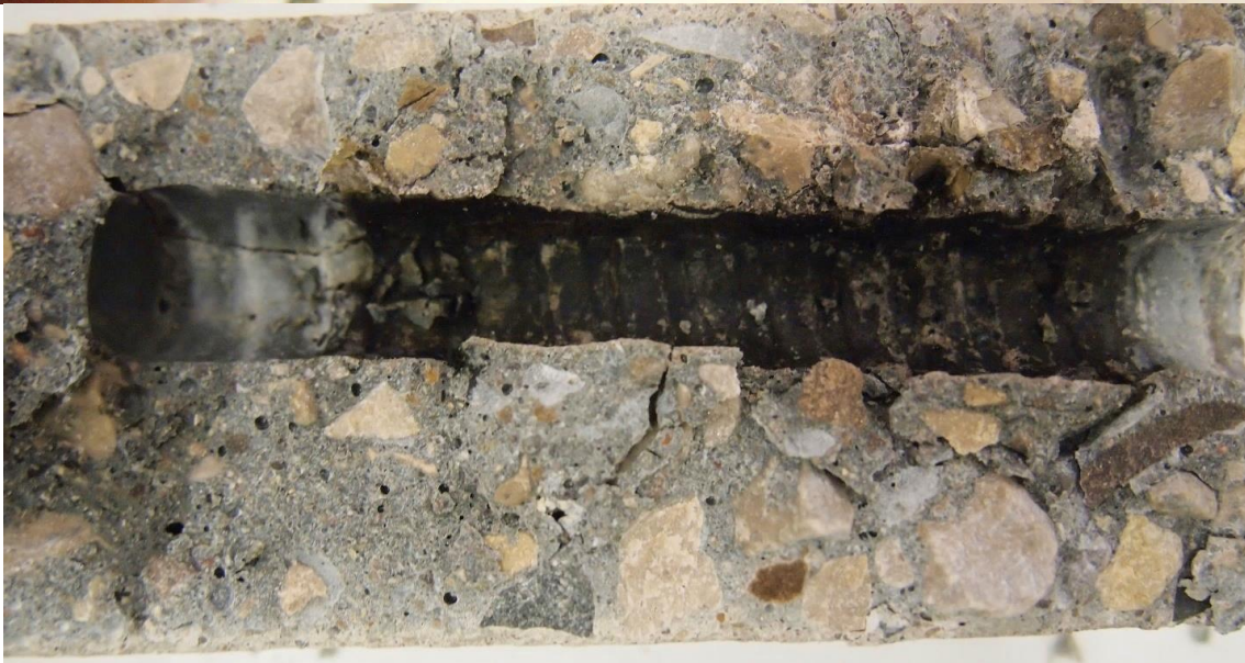
Figure C-22: Specimen SBO-06 before testing (top) and after testing (bottom). Corrosion product observed on rebar and on concrete surface in contact with rebar
