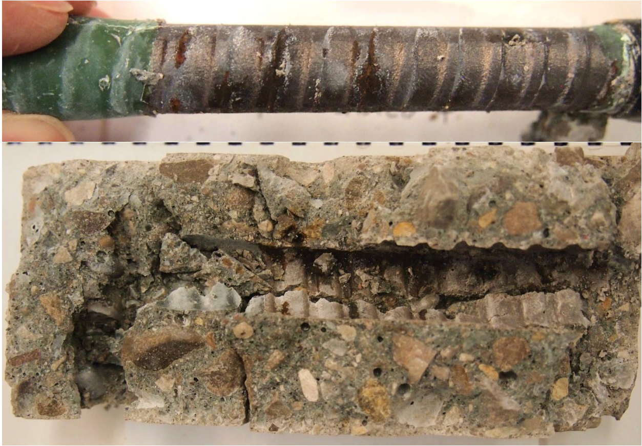
Figure C-19: Corrosion product observed on SBO-04 (top) and (bottom) some corrosion product observed on concrete
