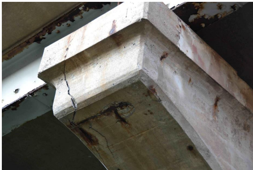
Figure 1-2: Corroded rebar causing cracking and spalling of concrete on a bridge pier [5]
