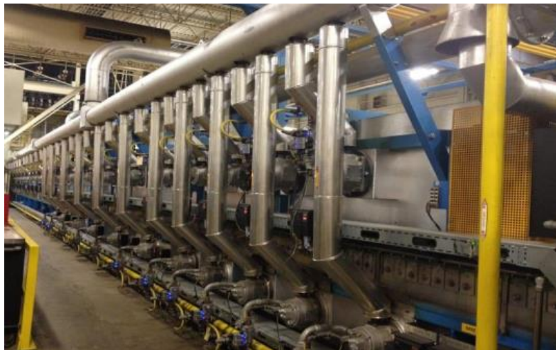
Figure 3: Roller hearth furnace at Formet Industries [19].
