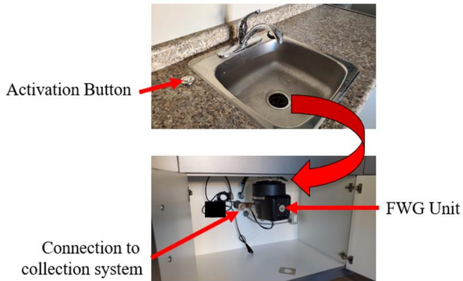
Figure 2. FWG Sink and Sink Arrangement in Standard Study Building Unit
