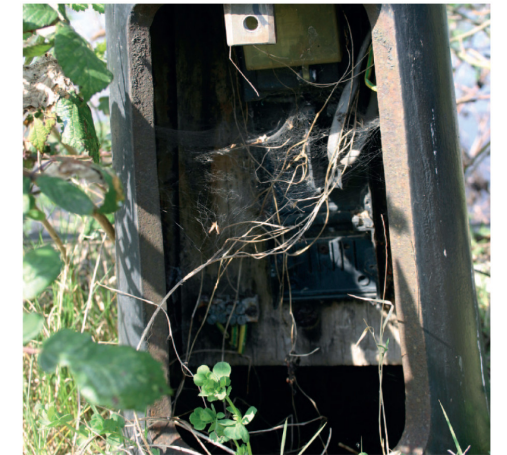
Figure 3. Web/sites. Plants, spiders and electric wiring in an old lamppost on the promenade of Pomona Strand, 4 April 2019. © Photograph: Emma Fraser and Clancy Wilmott.
