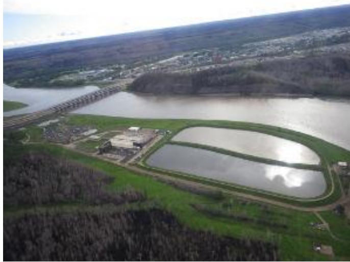
Figure 6: Regional Municipality of Wood Buffalo water treatment plant and Athabasca River (photo credit RMWB)
