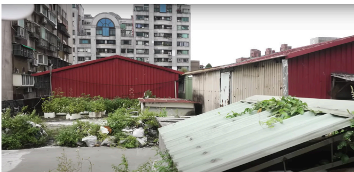
Fig. 1.33 Metal shed roof top expansions built mostly by the residents living on the top floor of the Xinwei Building.
