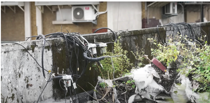
Fig. 1.34 Tangled wires can be seen on roof and throughout the facade of the Xinwei Building as an example of how electricity has been distributed.
