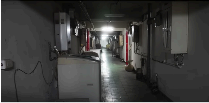
Fig. 1.32 Communal corridor filled with washer dryers, pipes and wires, and hot water tanks.
