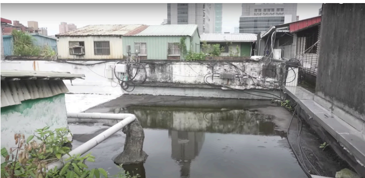
Fig. 1.30 The rooftop of the Xinwei Building. Electricity and water pipes are distributed to the illegal metal shed households.
