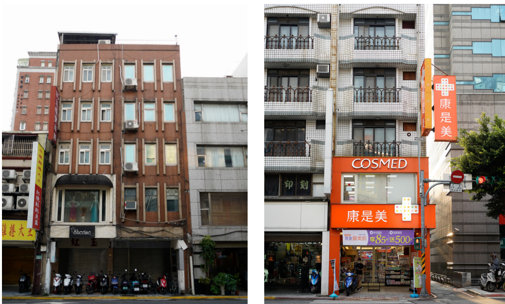
Fig. 3.62 Two of the shops on the project site occupy multiple levels of the streethouse. The landlord of the "COSMED" pharmacy shop has removed the concrete stair core from its original location and moved it to the back of the building in order to expand the commercial space.
