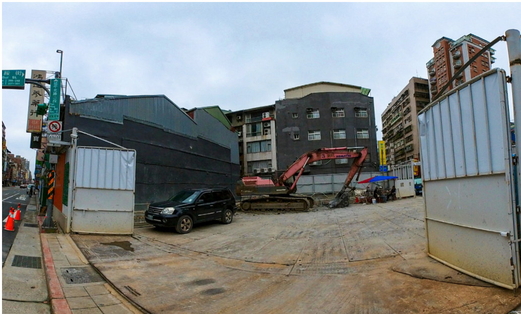
Fig. 3.40 The demolition site at the intersection of Guisui Street and Section 2, Yanping North Road.
